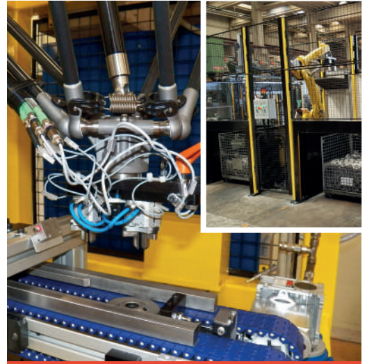
Robot loading from bulk containers.
